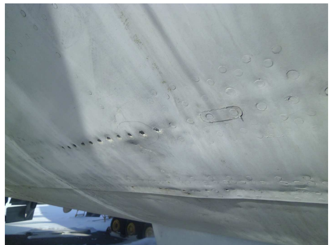
Fig. 1. Failures of TU-154 riveted joints
