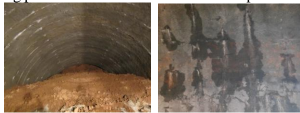
Fig.2 Leakage situation of primary support
