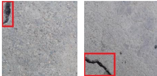
Fig. 2 Pictures of crack at four edges
